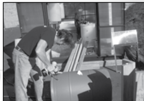
Pictured are Mr. Christopher Hartmann and KHS student John Smialek installing hydroponic tanks in the new greenhouse.
